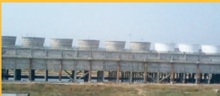
SUPER THERMAL POWER PROJECT AT NAGPUR, MAHARASHTRA
